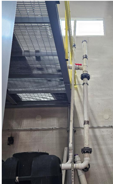
Figure 2 - Big - 1150 Vent Stack
